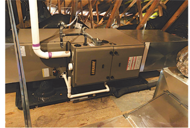
Closeup of new HVAC equipment
