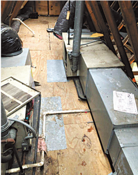
Old HVAC installation
