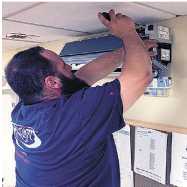
Paradigm Project Manager Richard Nimmo installs the iWave-M on the Fujitsu wall head.
